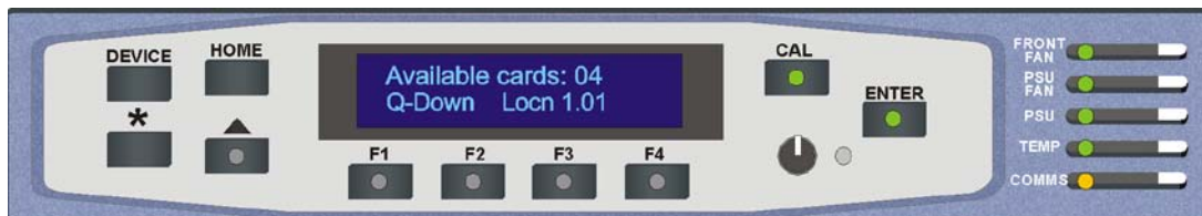
Control panel showing available cards
